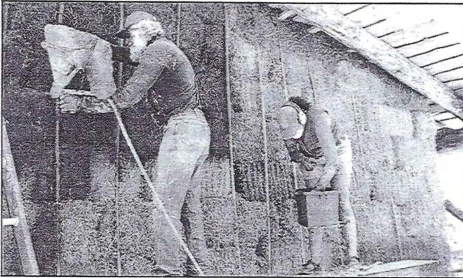
The exterior straw bale wall of this Build Here Now structure is held together with bamboo (rather than rebar) on both sides of the wall, which are tied together through the bales. This wall is being prepared for mud plastering.
