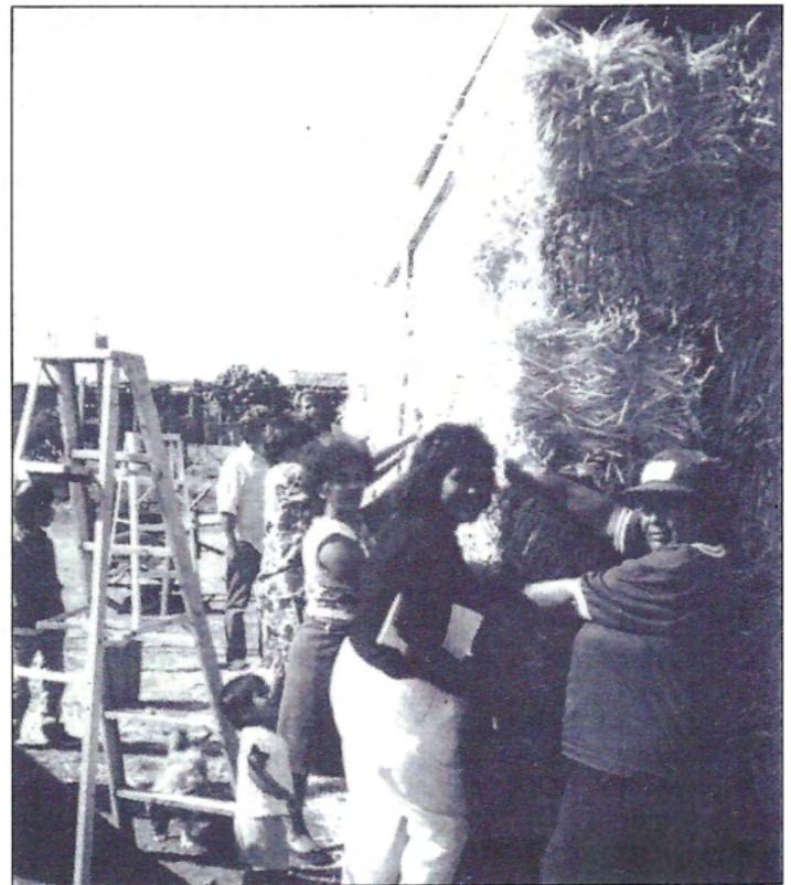
Mexican villagers learn from Farmer-to-Farmer volunteers how to convert agricultural waste products into efficient and affordable housing.
